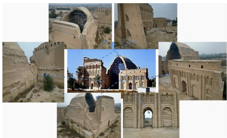
Figure 4. Current-condition field documentation of Taq Kasra showing detailed views of the vault, cracked and leaning walls, brick coursing, and facade elements at multiple locations across the site, referenced against the overall elevation. Source: Alzubaidy [5].
